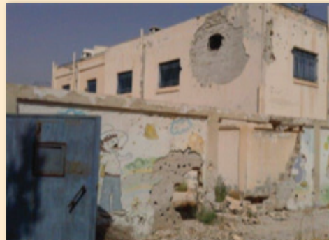
One of the damaged UNRWA schools
