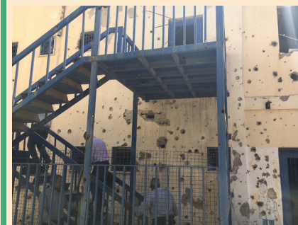
Damaged health centre
