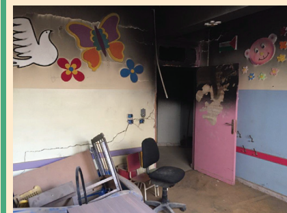
Damaged kindergarten in community centre
