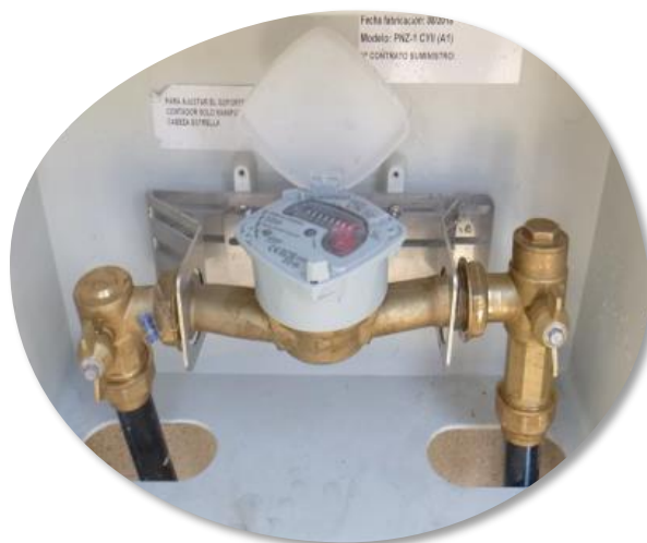
Figure 3: Water meters in isolated arrangement
