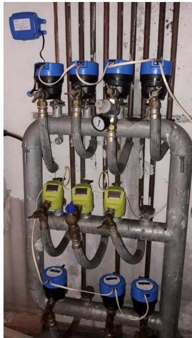
Figure 5: Distribution of electronic water meters in bus UNE-82326:2010 and NB-IoT concentrator
