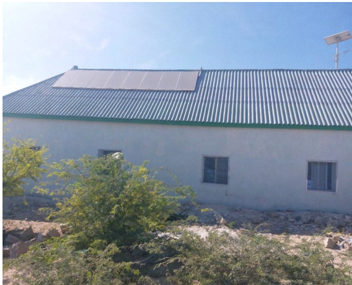
Figure 10: Solar panels at Hobyo Community Social Centre
