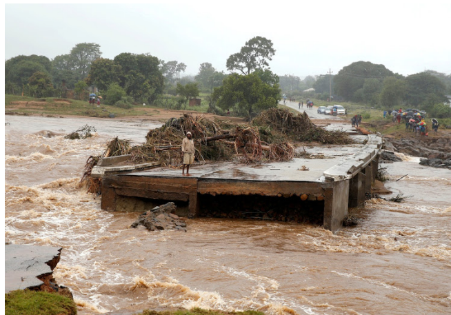
Figure 4-3: Washed away bridge in Zimbabwe due to Cyclone Idai
