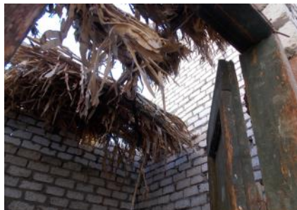
A decayed rooftop in the Baskaloun Village (El-Edwa, Minya) in need for restoration
