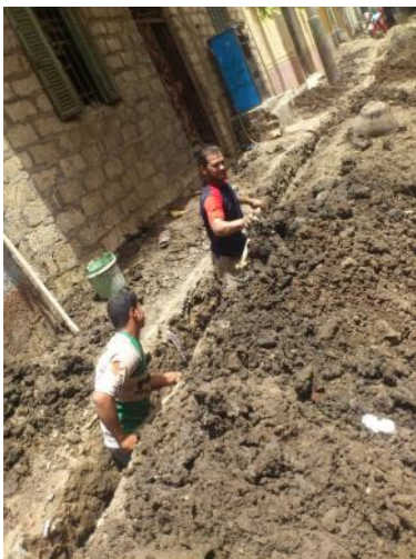
Workers laying pipes for the drainage canal newly constructed by HAYAT in El-Sawy Village, Edwa
