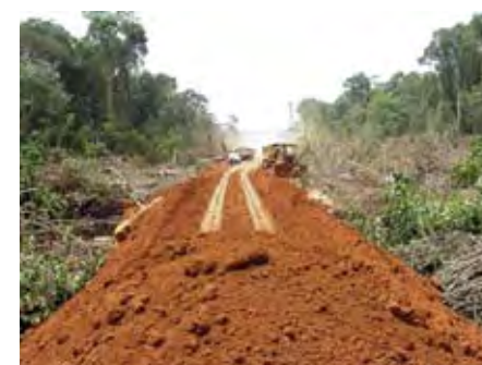
Road constructed through swamp forest to reach the Loudougou concession in northern Congo. Photo by Nadine Laporte.
