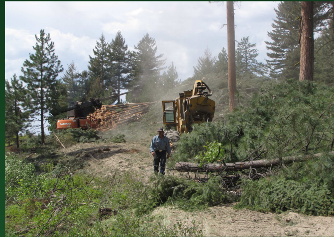
Thinning ponderosa pine under a stewardship contract on the Bitterroot National Forest in Montana.
