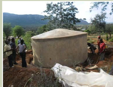
New water tank at Makwasinyi (Oct 2012)
