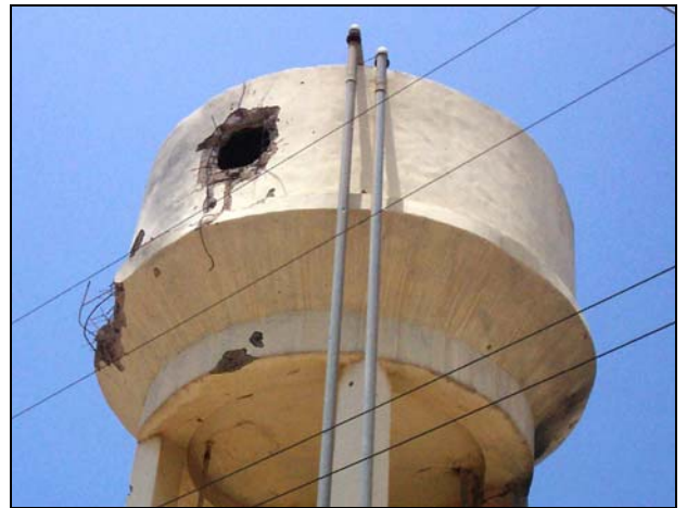
Water tank damaged in Nahr el-Bared
