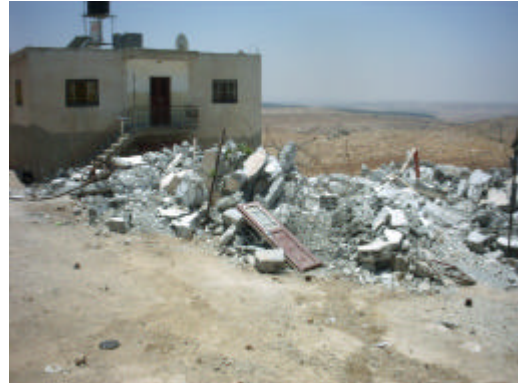
Below and left: Homes destroyed near Eshkolot settlement
