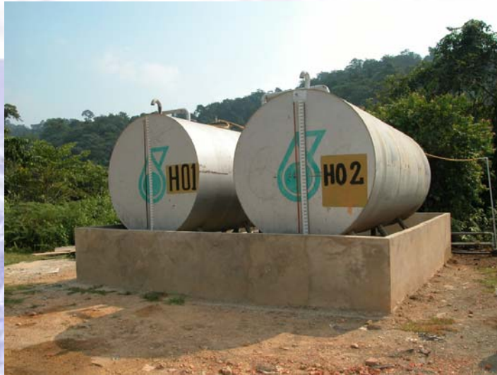
Containment bund for fuel tanks
