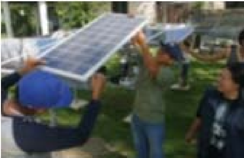
Installing solar panels for electrifying remote villages in conflict ridden areas of Mindanao
