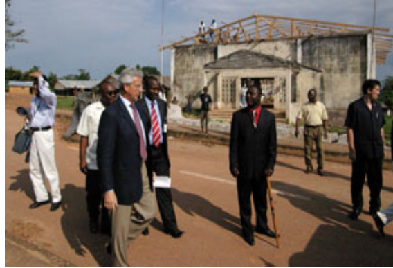
DSRSG da Costa and Superintendent Christopher Bailey visit the Circuit Court currently under construction through UNMIL’s Quick Impact Project.
