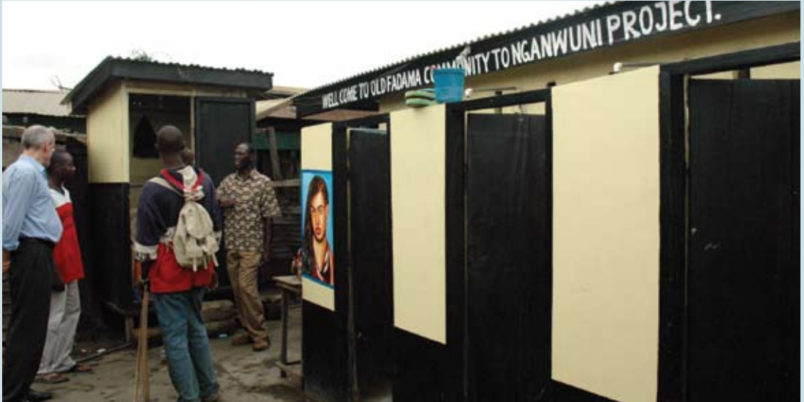
UN-HABITAT focus: Environmentally sound basic urban infrastructure and services - a new shower block for women and men with clean running water in a slum in Ghana. Photo ©: UN-HABITAT/S. Mutter
