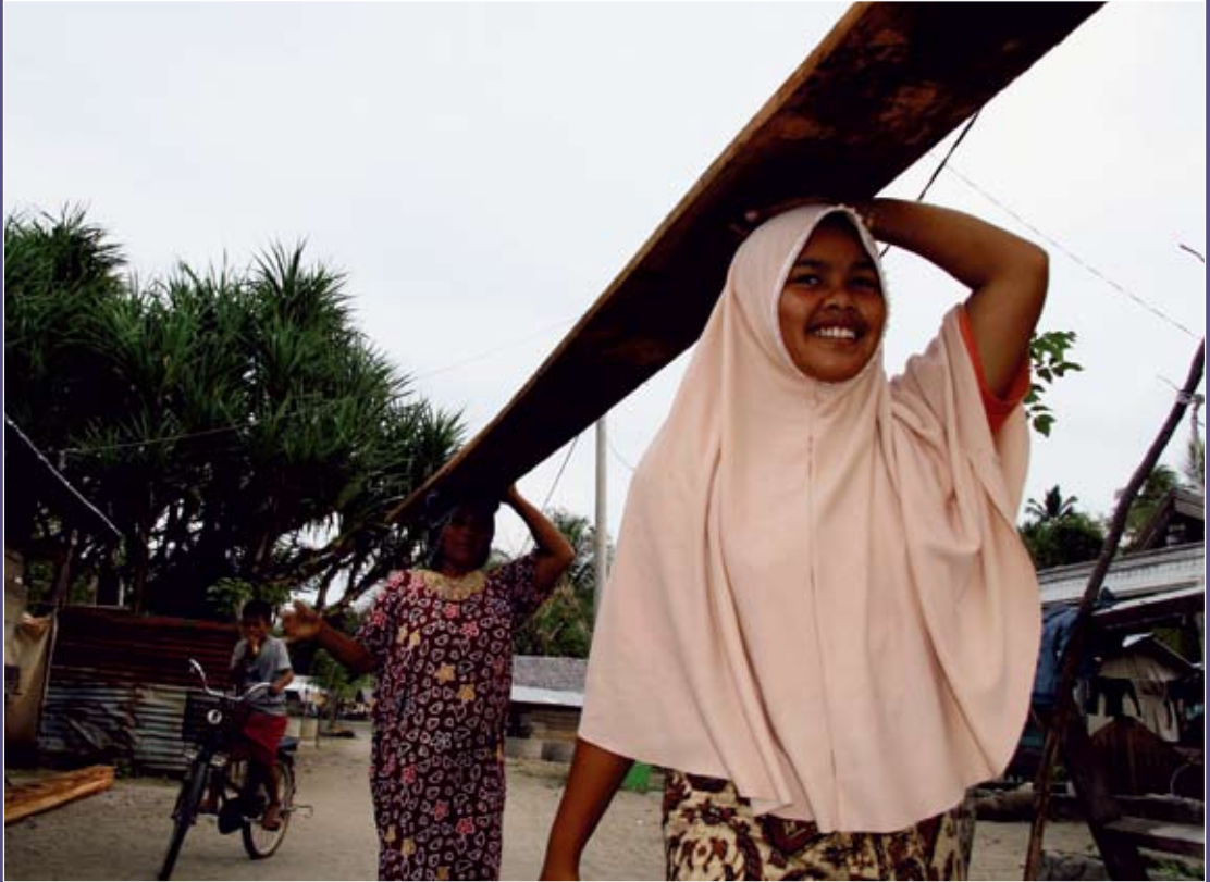
Rebuilding after the destruction wrought by a tsunami killer wave in Banda Aceh, Indonesia. Photo © UN-HABITAT
