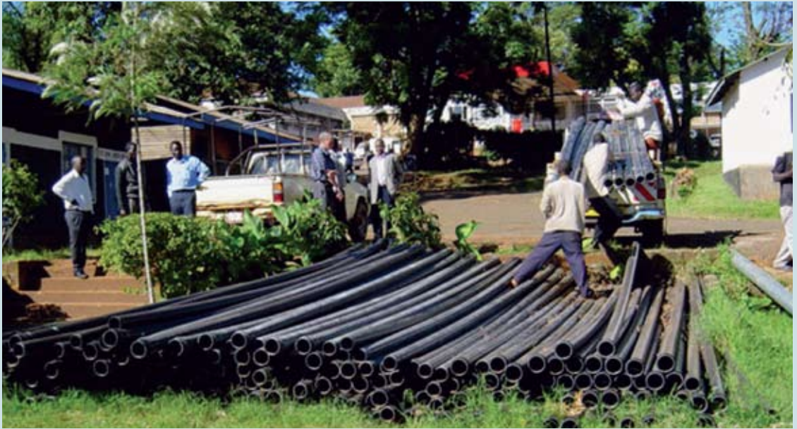
Contractor delivering pipes for a water project in Kisii, Kenya. Photo @ UN-HABITAT
