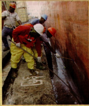
WORKERS of Tiger Tanks, the company hired to conduct mop-up operations regarding an oil slick in the Gulf of Paria, scrub oil from the cargo vessel Fabian Schulte yesterday at the Port of Port-of-Span, where it was berthed. PHOTO BY AZLAN MOHAMMED
