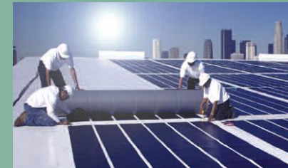
Integrated Solar Roofs
