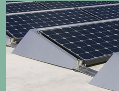
Solar Roof Array
